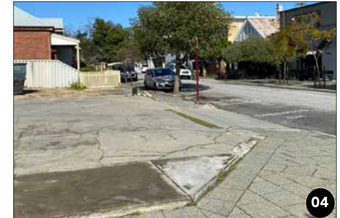
04 The lack of trees and landscape would increase the heat island effect.
