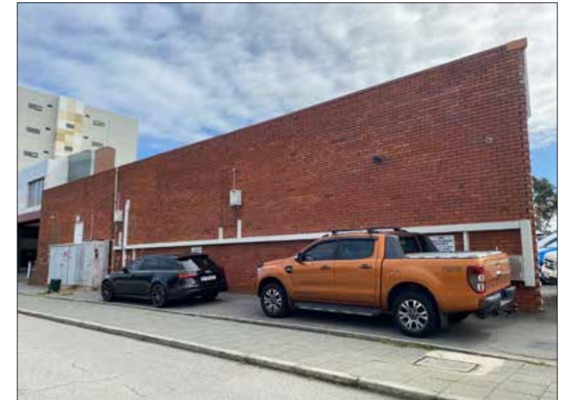
The blank facade creates an uninviting pedestrian environment.
