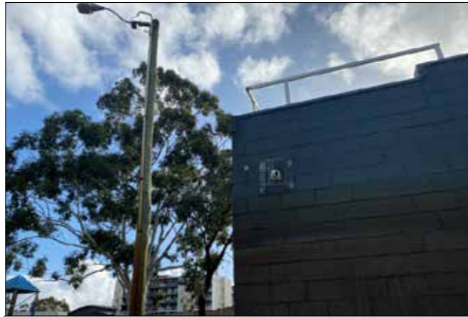
Lighting and CCVT camera.
