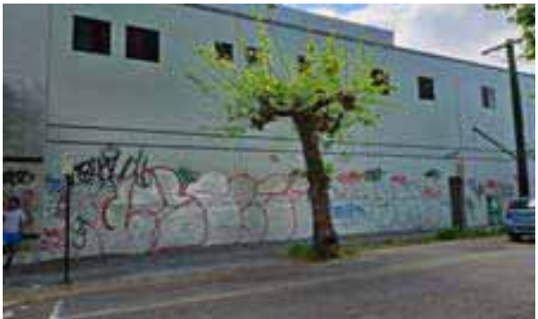
Graffiti covered wall
